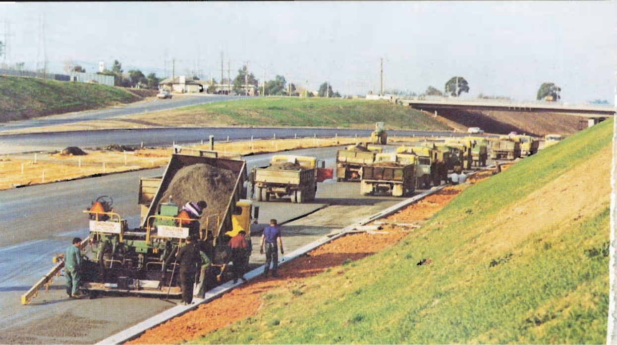
Asphalt sealing in progress on the Mulgrave Freeway, July 1976. Country Roads Board
