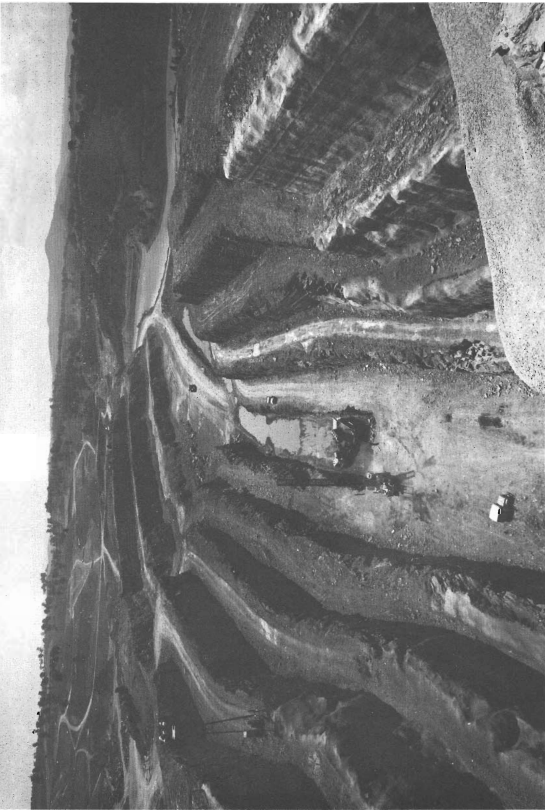
Excavation for the draw-off channel which will convey water from the Sugarloaf Reservoir in the Christmas Hills area for delivery to the water treatment plant.
