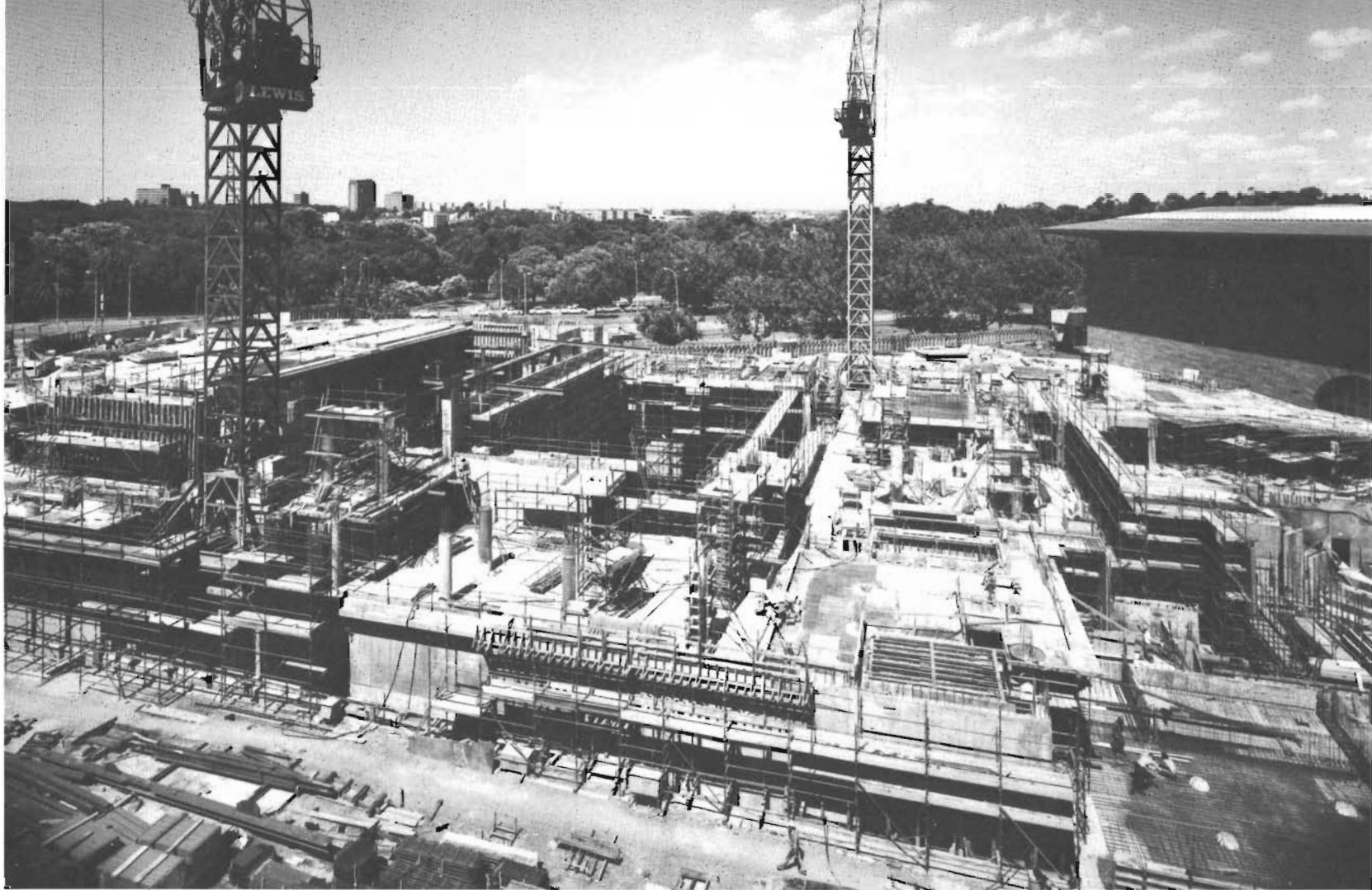
Work in progress on the Theatres building at the Victorian Arts Centre during December 1978. The view is taken from City Road, South Melbourne.
