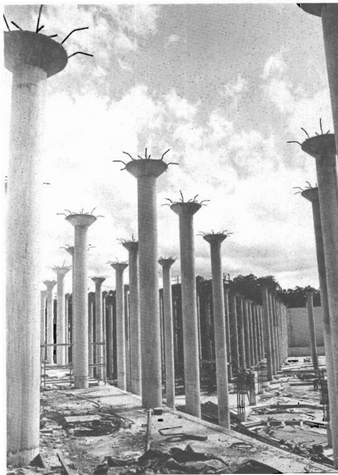
Support columns for the roof of the Sugarloaf Reservoir clear the water storage which will have a capacity of 200 megalitres.
